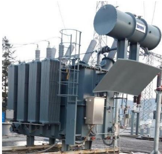
Figura 3 - TR 18EN084 25/25/8 MVA, TTOE
