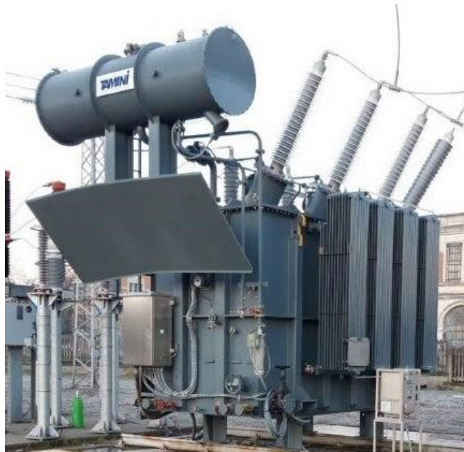
Figura 1 - TR 18EN084 25/25/8 MVA, TTOE
